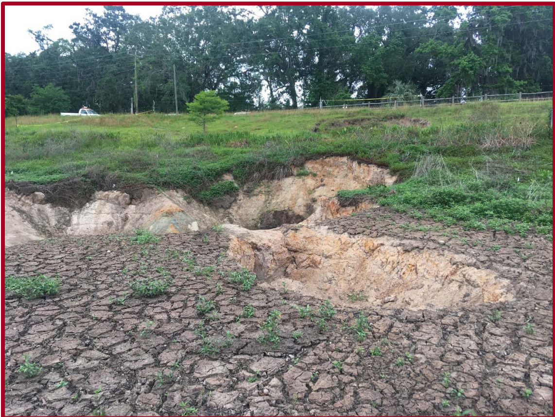
FIGURE 3D: PHOTOGRAPH OF EXISTING SITE CONDITIONS NEAR SOIL BORING VB-17 (FACING WEST)
